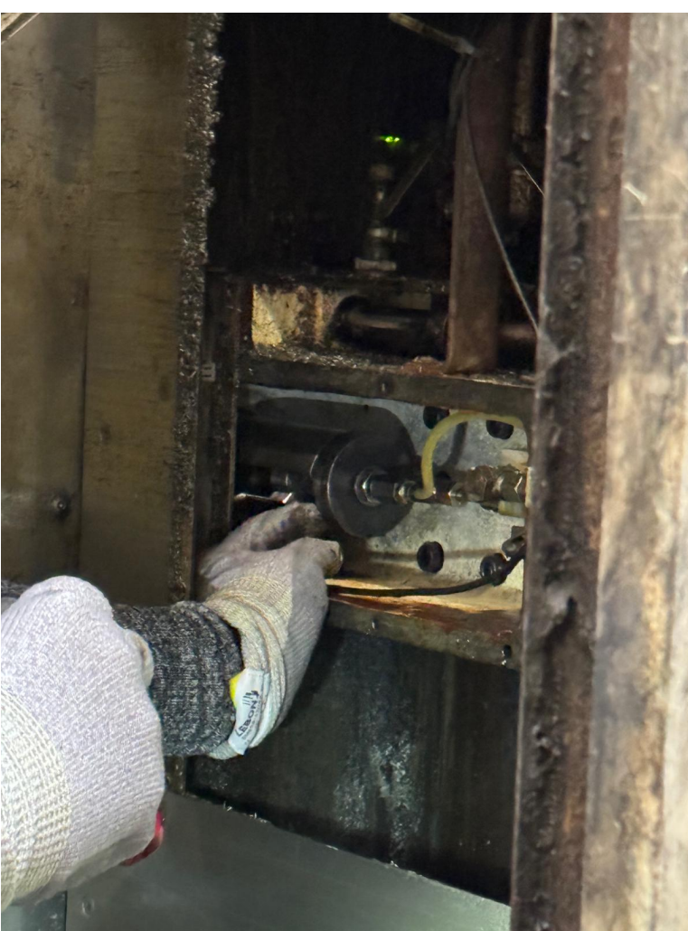
Image 13. Working on the sensor mentioned above, inside the machine.
