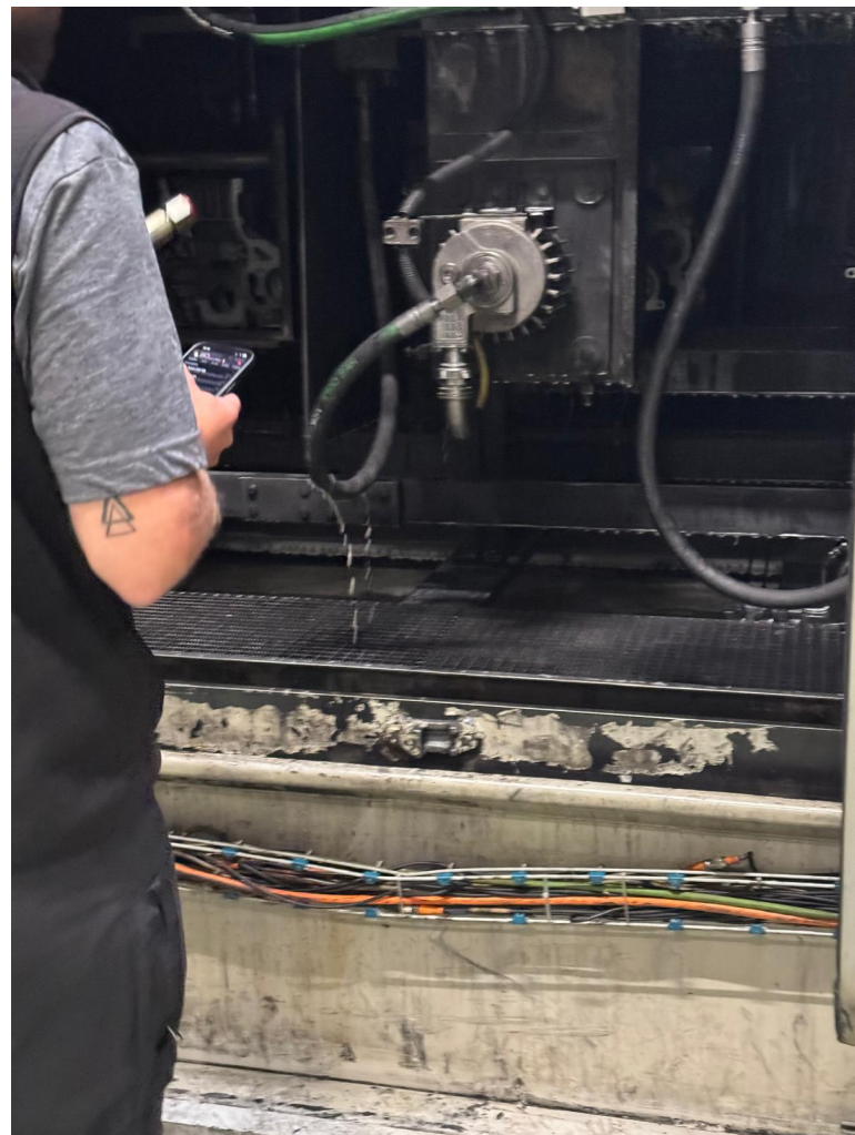
Image 16. The leak on the washing machine hose mentioned above, located at a fitting.
